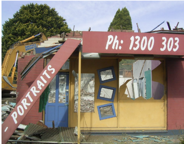
Demolition of the buildings from the converted Coach & Horses Hotel on 4th May, 2005
